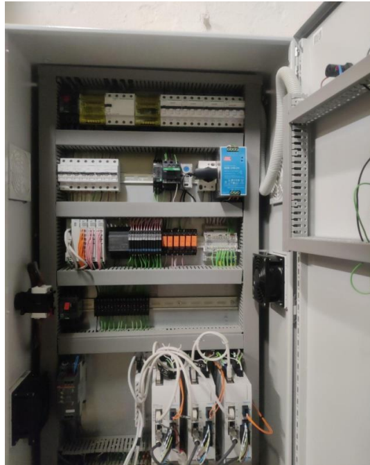
Figure 15. The electrical cabinet that enables the operation and control of RoReWos and their integration with the rest of the prMRF components.
